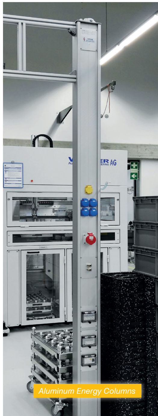
Underground distributors PIAZZA
